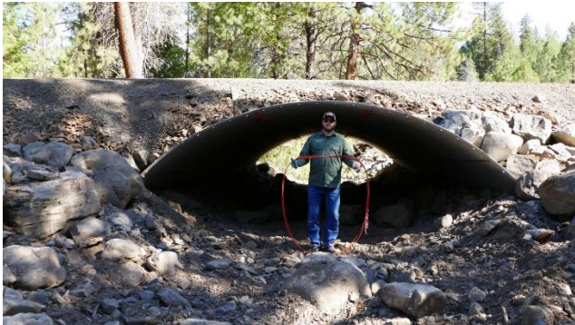
The orange rope represents the size of the previous culvert that was replaced
