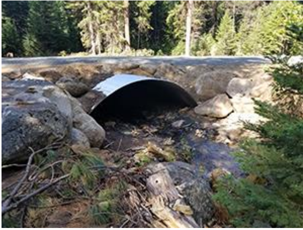
A new culvert installed on Deadwood Creek in the Malheur National Forest by the John Day Screens Shop using GNA
