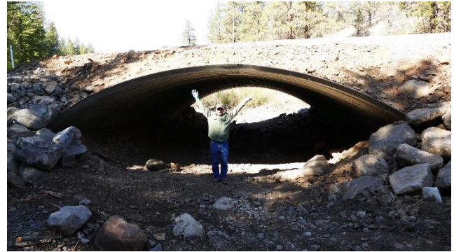
New thirty-three-foot wide, open bottom culvert that replaced two, six-foot wide culverts
